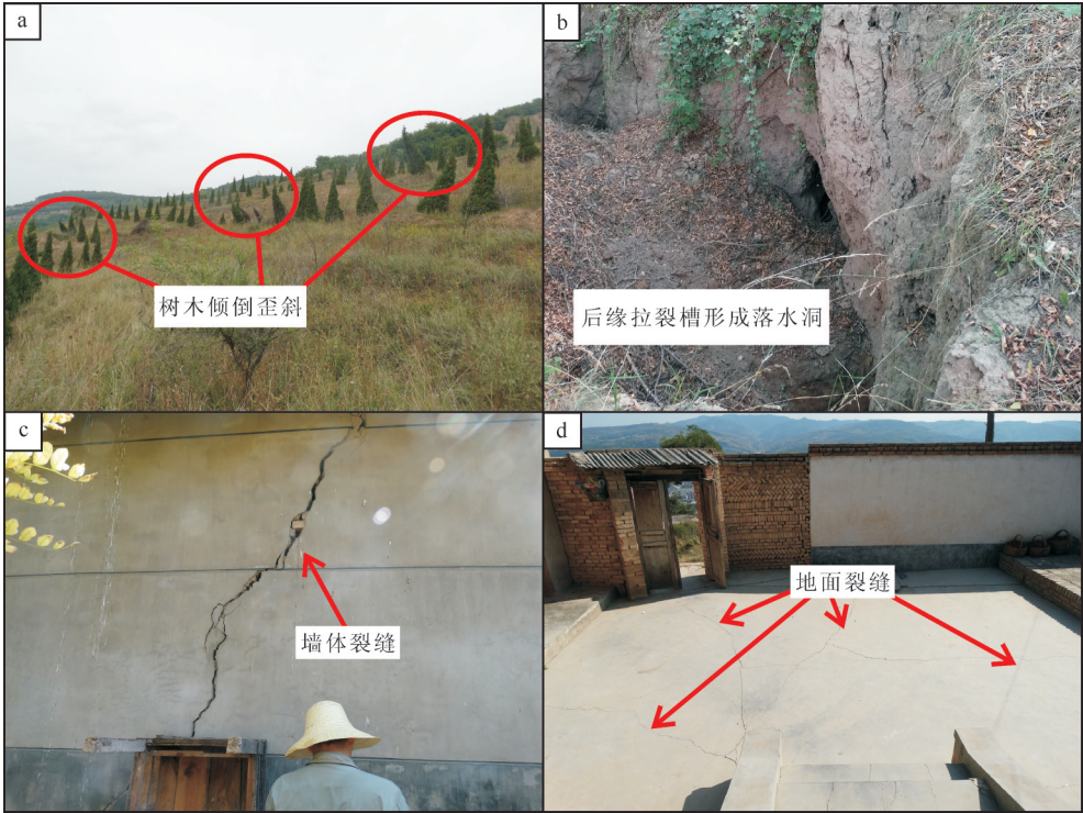
图8 红旗山滑坡现今变形破坏现象 a—树木发生倾倒歪斜;b—滑坡后壁发育拉张裂隙;c—民房墙壁出现剪张裂缝;d—民房地面出现拉张裂缝 Fig.8 Deformation features of Hongqishan landslide at present a-Trees falling and skewing; b-The development of slip cliff tension cracks; c-Shear cracks appearing on the house wall; d-Tensile cracks appearing on the house floor
